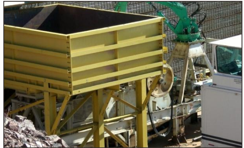
Jaw crusher & feed bin
