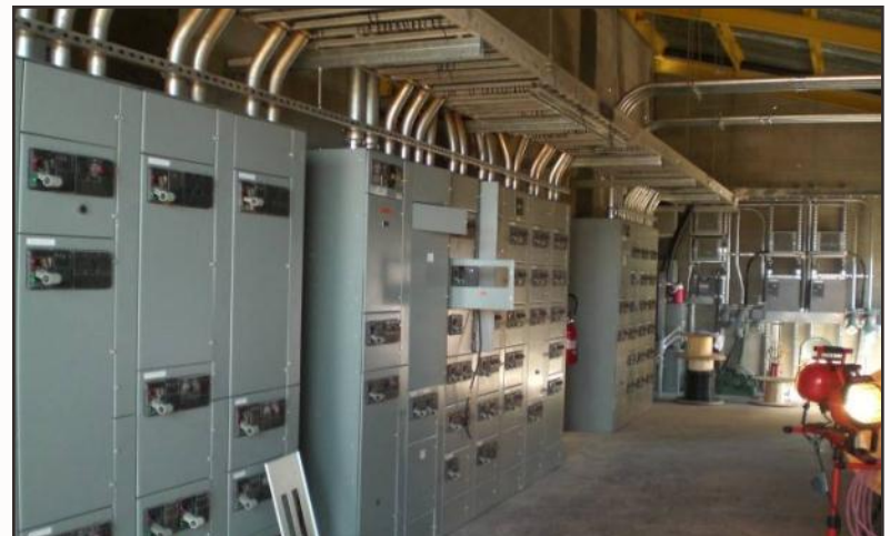
Electrical control room
